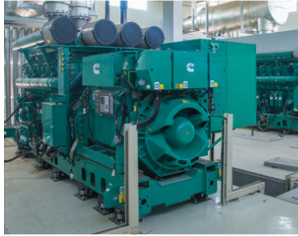
Two QSK95 units power the plant's high-capacity blowers
