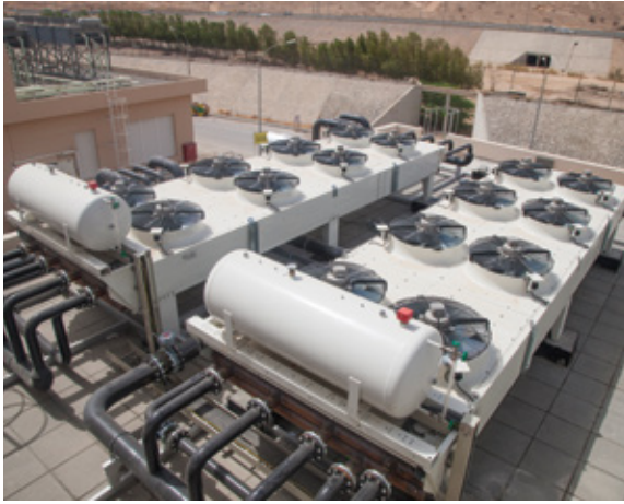
Remote radiators for the biological treatment plant
